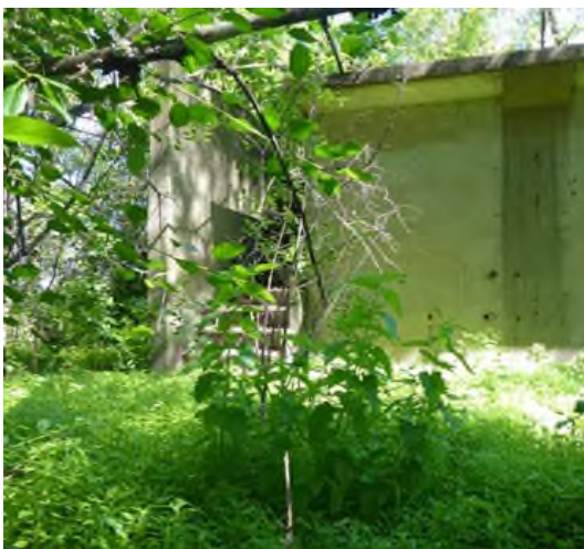
Fall Hazard: Steps leading to an unprotected second level
