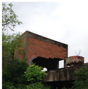
Structure at risk of collapse
