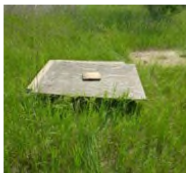
Covered holes and pits
